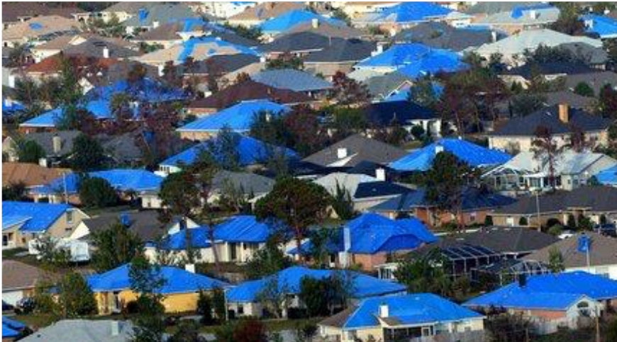
Figure 1. Blue tarps on roofs after hurricane [6].
